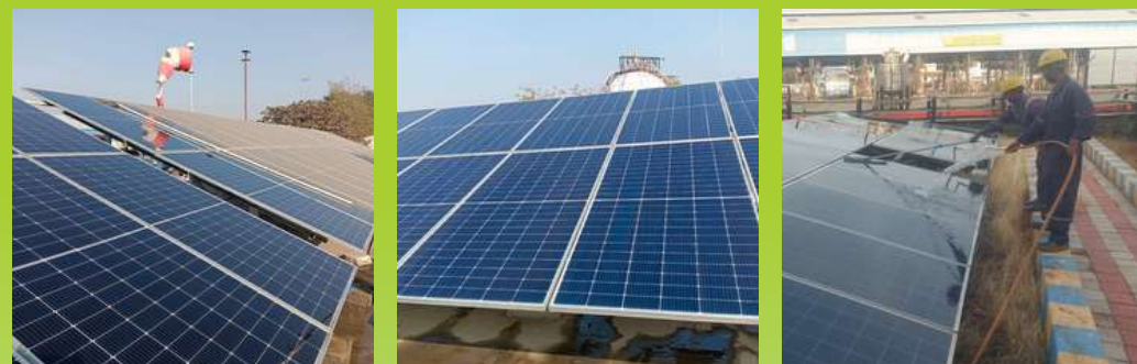
Bharat Petroleum Corporation Ltd. 4540 Kw & 4125 kw
